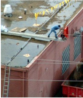
Safety Photo of the Month!
