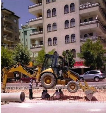
Safety Photo of the Month!
